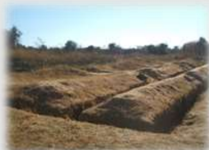
What was field space behind the school is now being prepared for new classrooms
