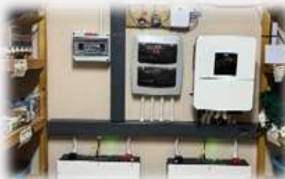
The system has 2 large batteries charging from solar and Zesco
